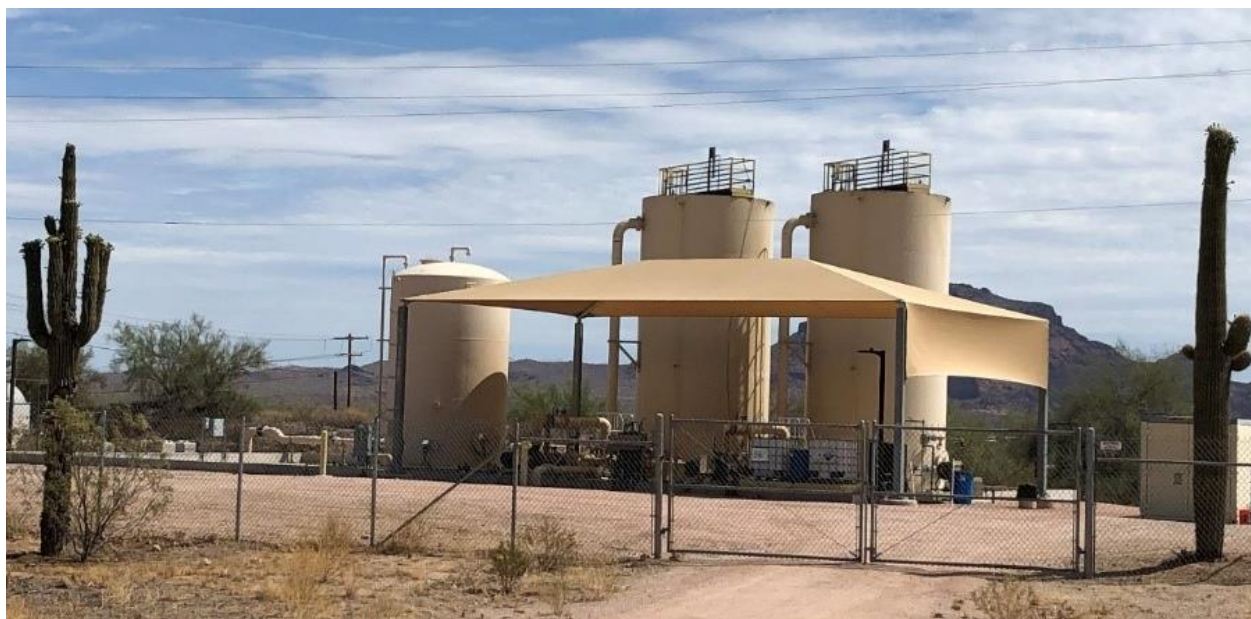
Figure 4 (Photo) – FBR Groundwater Treatment System
